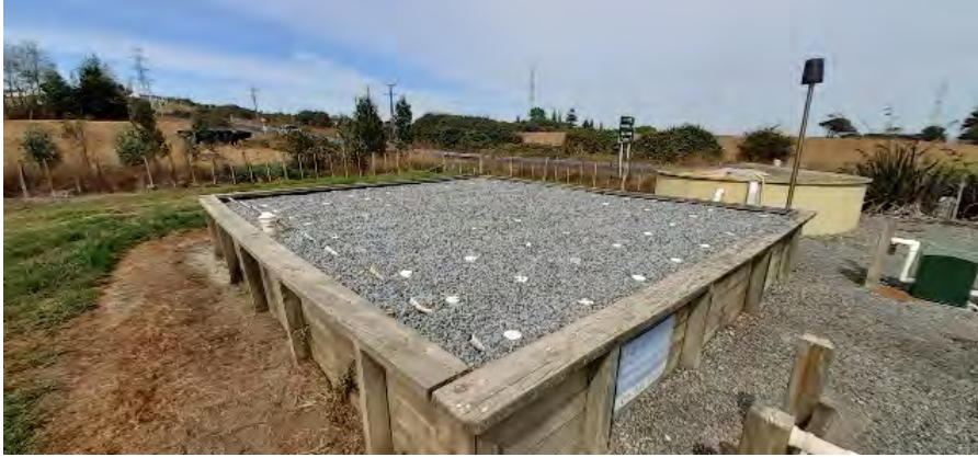
Maramarua WWTP after media replacement
