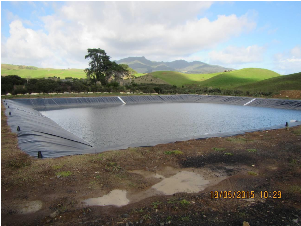
Newly commissioned sealed final effluent holding pond
